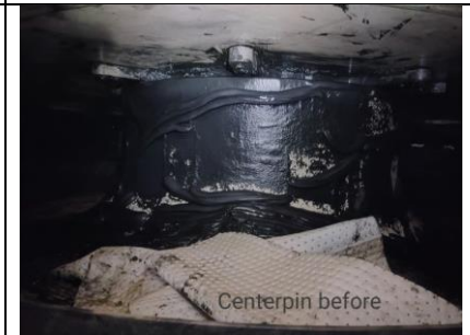
k. Clean grease removal from centre pin area pathways, floor, and roof with degrease clean
