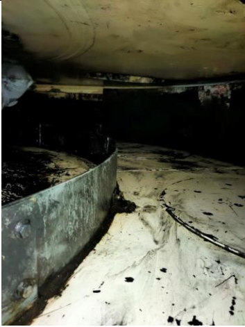
k. Clean grease removal from centre pin area pathways, floor and roof with degrease clean
